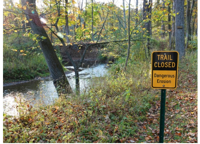
Unfortunately, some trails had to be closed due to erosion
